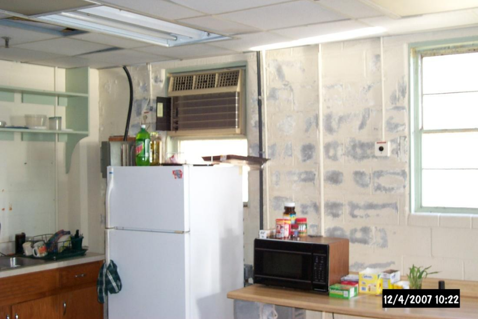
Moisture Bleeding Through Interior Walls
