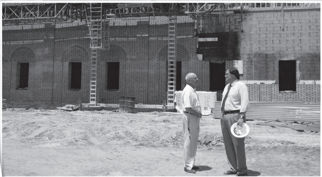
Jimmie Laycock and W&M President Gene R. Nichol look over the Laycock Center construction.
