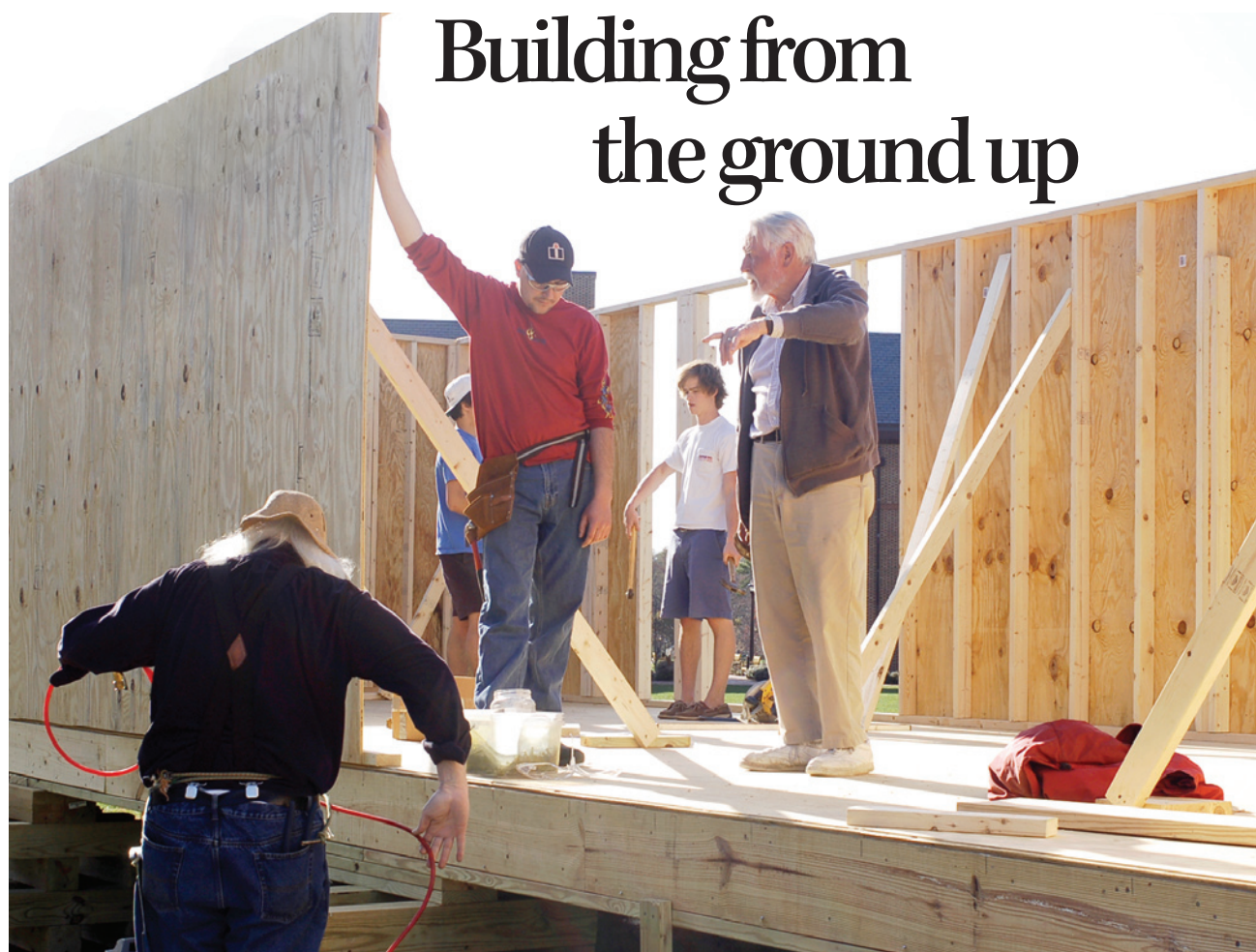
SUN PARK — THE FLAT HAT Volunteers with the Williamsburg Housing Partnership, Inc. plan to finish construction of a house on Jamestown Field by April.
