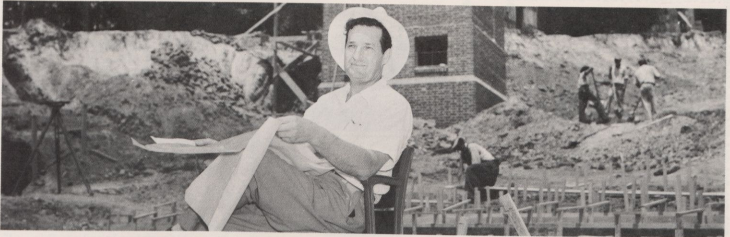
Paul Green, author of The Common Glory, overseeing construction of amphitheatre in 1947.
