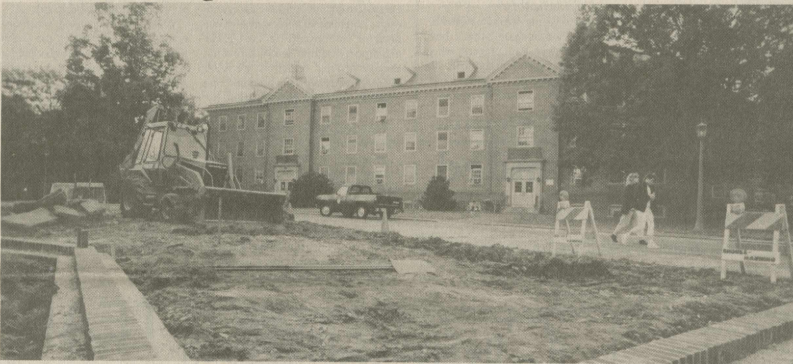
Construction on parking for Blow Memorial Hall began this week. The lot should be ready by December, when the building is set to open.
