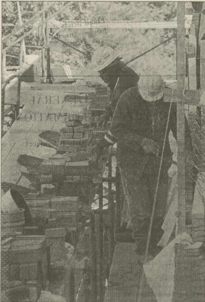
CLOCKWISE FROM TOP LEFT: (1) Bricklayers work to finish the outside of the Swem addition. (2) This metal stud framing will form a portion of the special collection wing's roof. (3) When completed this will be the passageway between the current Swem building and the new renovation. (4) Construction worker Tyrees Kelly, who is a pre-law student at Norfolk State, takes a lunch break. (5) The construction work is now primarily focused on exterior work. Beginning next August, the focus will shift to interior areas, such as this. (6) Using a specialized saw, a worker cuts pegs for steel beams.
