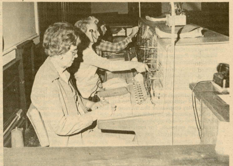
William and Mary telephone operators Ann Whittaker, Hazel Sych and Sam Spalone expect next week to be hectic, while the campus adjusts to the new centrex system. The current switchboard will be replaced by two modern push button consoles.
