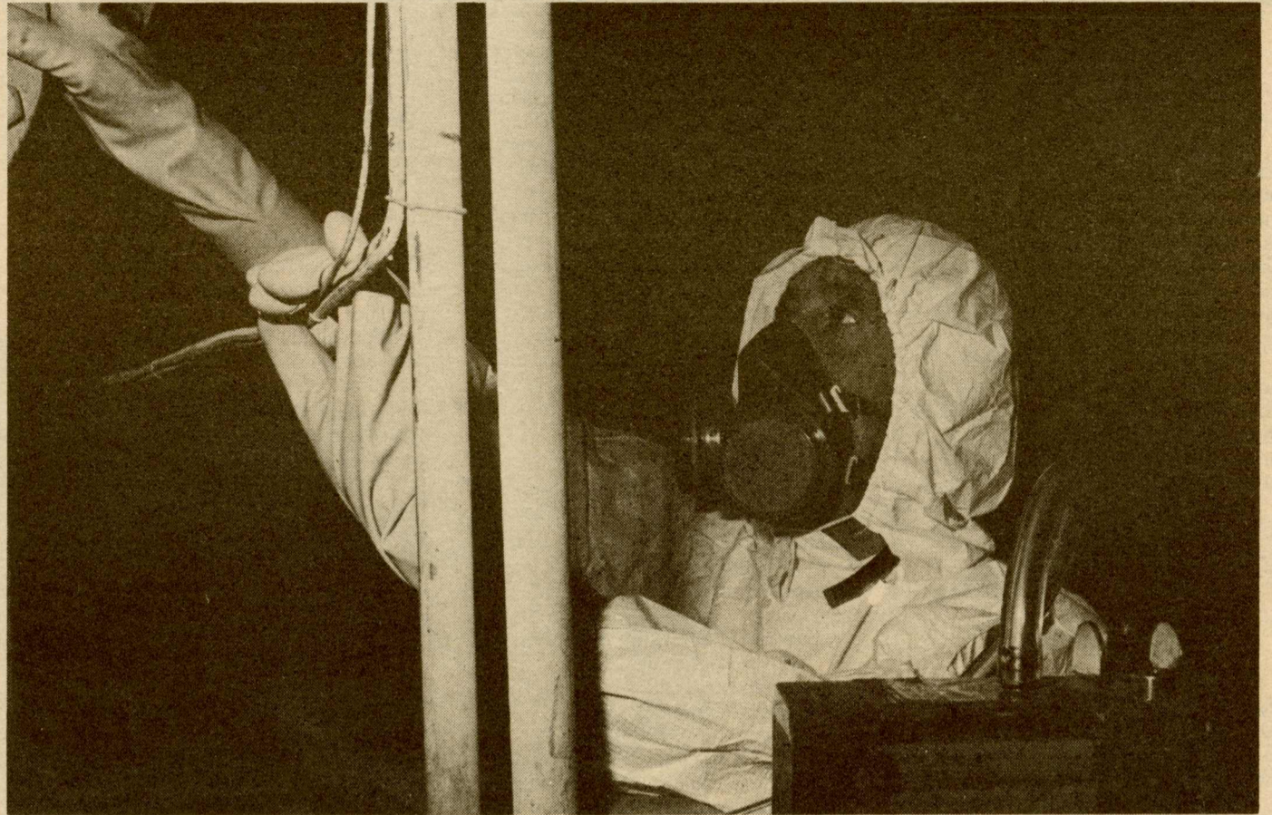
Bob Jordan, industrial hygienist and consultant for the asbestos removal project at the College, uses a sampling pump to check the level of asbestos fibers in the air in the basement of Millington Hall. In the background is Danny Dobbins, foreman for Spinazzolo Spray Systems.
