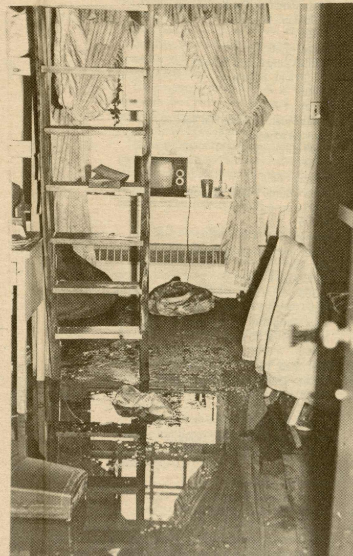
A second floor room suffered smoke and water damage but some items were saved.
