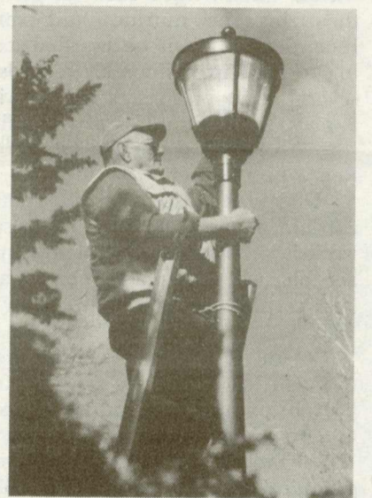
Electrician Don Morgan finishes replacing a light fixture in front of Phi Beta Kappa Memorial Hall.
