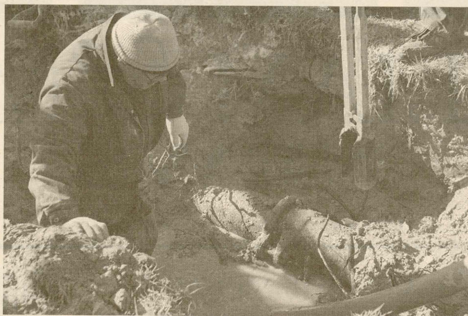
Chief plumber Edward Martin of facilities management repairs the rupture in the underground water pipe that burst last Wednesday evening near Ewell Circle.
