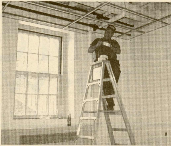
Construction will continue through the summer on new dormitory rooms in the Bryan Complex.
