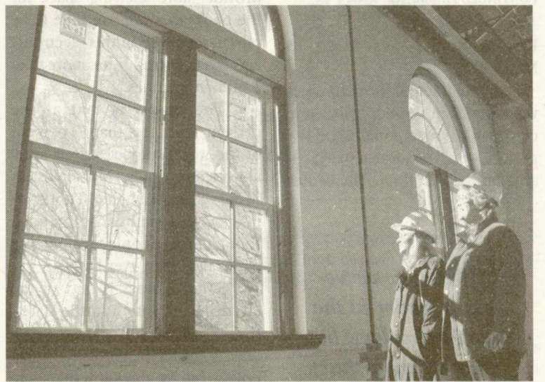
Ksenia Jaroshevich (l) and site manager Kay Van Dyke inspect the new, state-of-the-art windows that have been installed in James Blair Hall.
