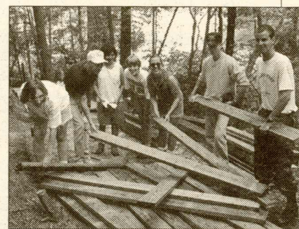
Law students built several new bridges for foot paths at York River State Park.
