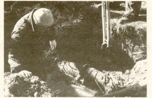
The new water line system will allow for the speedy repair of breaches like this with limited disruption of water service.
