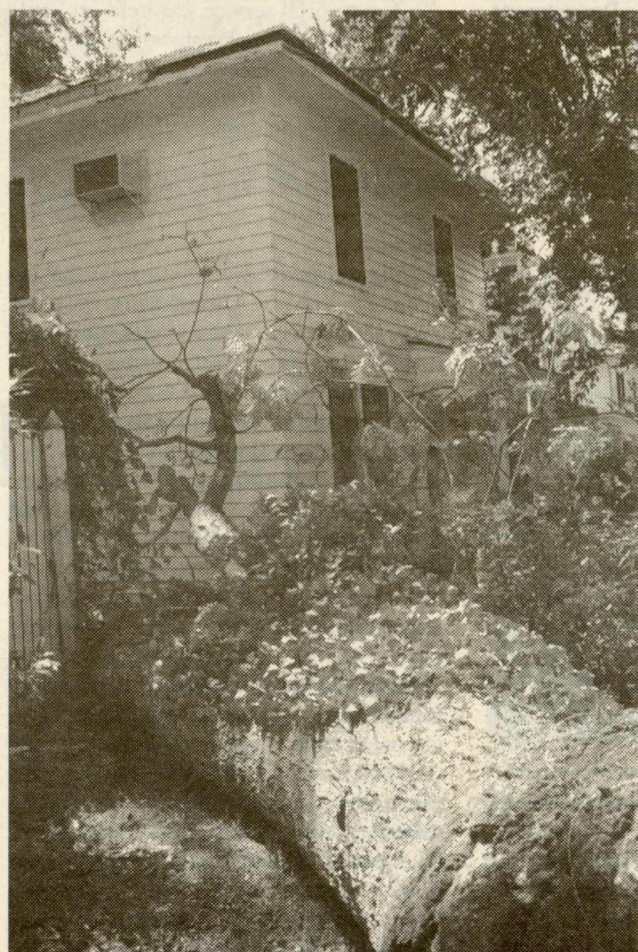
Holmes House on Jamestown Road suffered structural damage when a tree fell through a ground floor window of the building and destroyed a window air conditioner.
