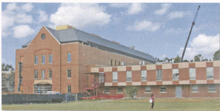
Construction of Phase I of the Integrated Science Center is nearing completion.
