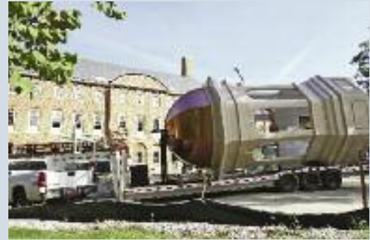
The 28-foot high cupola is readied for installation atop Alan B. Miller Hall, the new home of the Mason School of Business.
