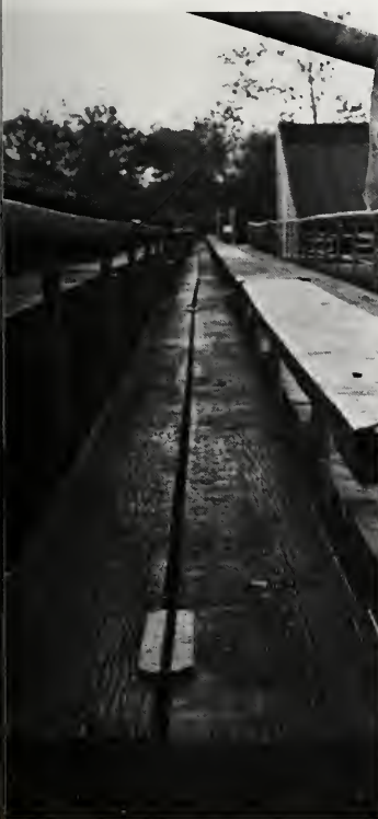
One phase of the expansion plans the removal of rickety wooden bleacher seats.
