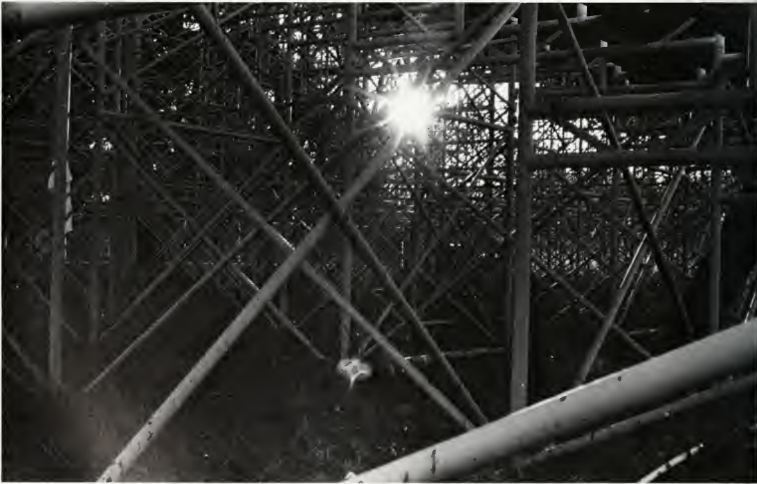
Highlighted by the setting sun, a maze of interwoven pipes supports the bleachers in the end zones.
