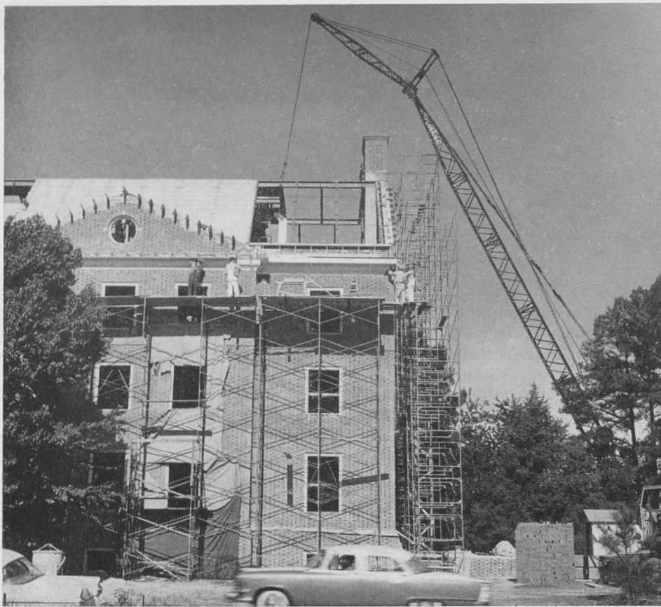
A new girls' dormitory rises beside Chandler Hall and overlooking the Lily pond. When complete it will house 217 students.
