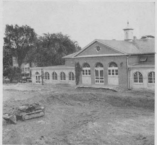
Pictured to the far right is the newly-completed Landrum Hall. The center spread is an artist's concept of the new Student Center; above is the excavation for this new building.
