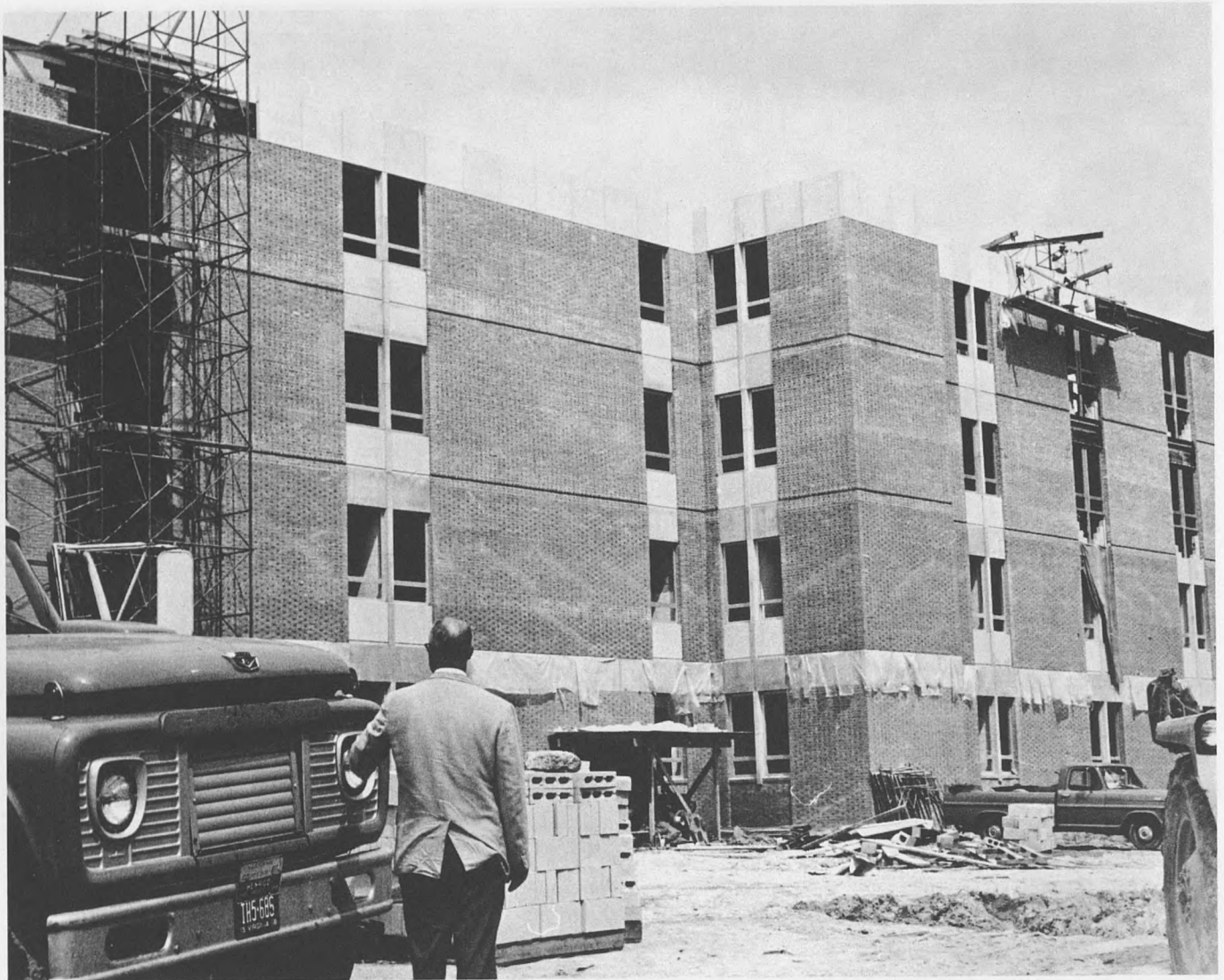
Dean Quittmeyer views construction of new Mathematics-Computer Center classroom building, to house School of Business Administration next year.
