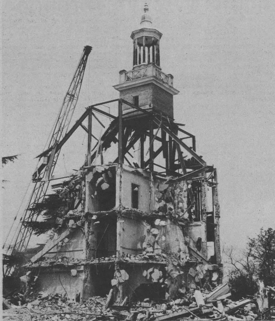
End of an Era — The final remnants of the old Eastern State Hospital Building near the William and Mary campus are fodder for the wrecking crane just before the destruction of the building is completed in April. For many years a landmark in Williamsburg, the building, located on property which now belongs to William and Mary, was removed to make way for the new National Center for the State Courts.
