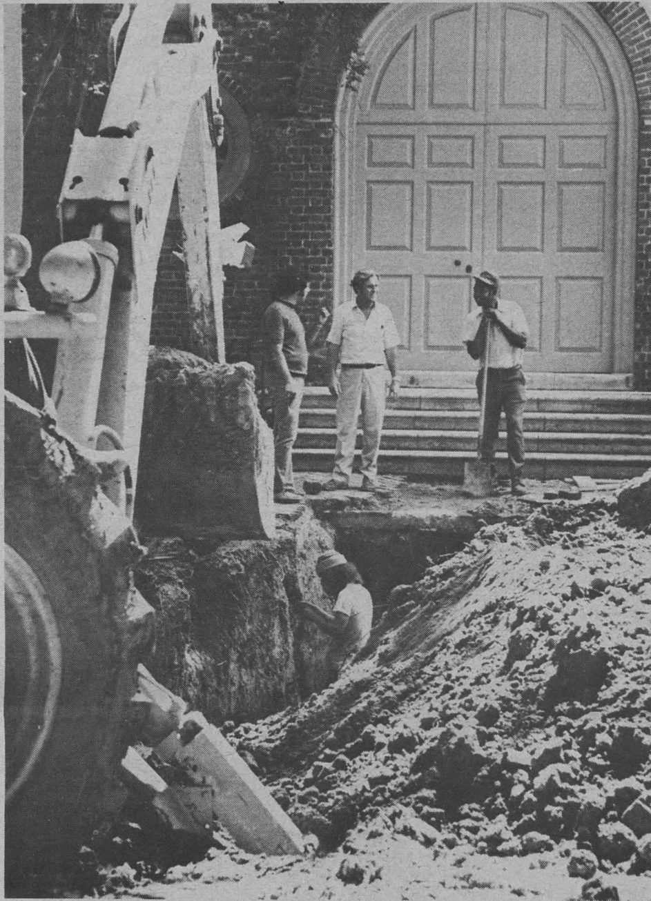
Workmen and archaeologists combine efforts to uncover the hidden foundation of the Wren Building.
