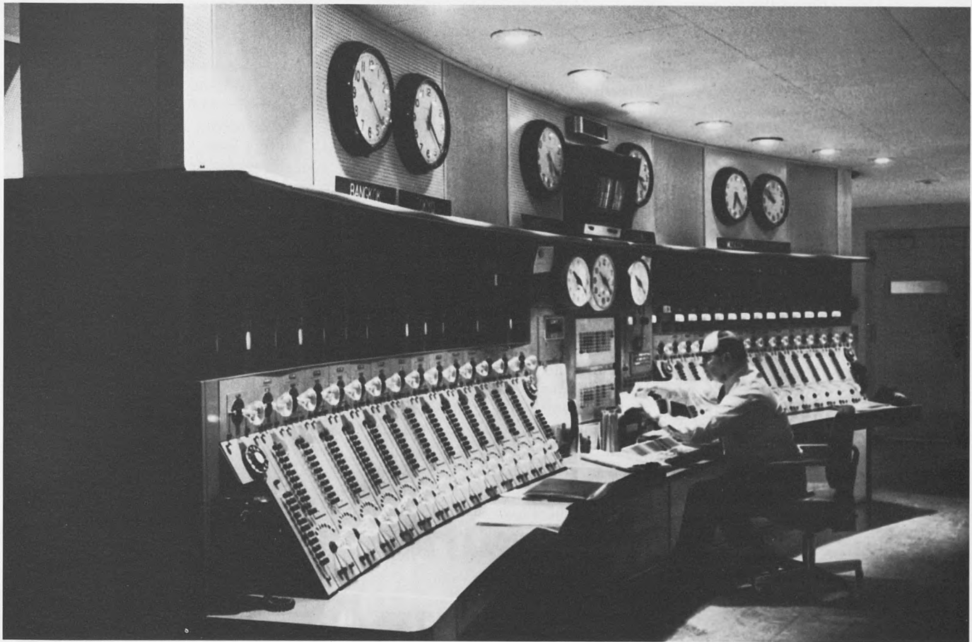
A control panel in the Voice of America headquarters links studios there with an estimated 80 million listeners around the world each week. VOA broadcasts 875 hours weekly in 39 languages.
