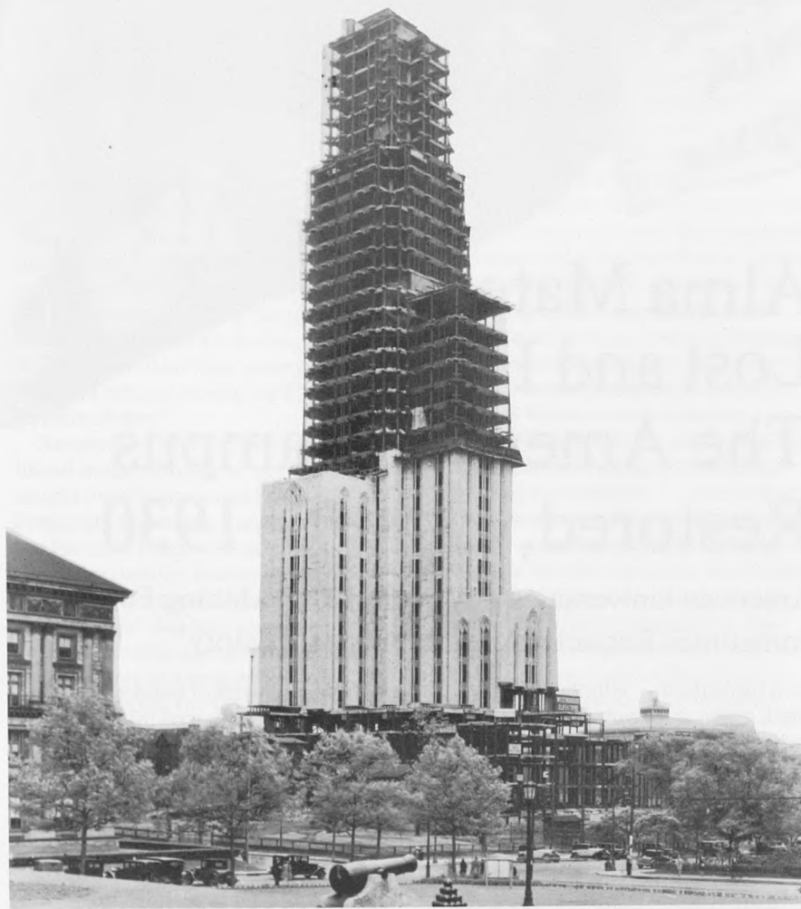
The mix of Medieval and Modern Forms in the University of Pittsburgh’s remarkable “Cathedral of Learning” (circa 1928). (Courtesy of the University of Pittsburgh Library, Department of Special Collections).
