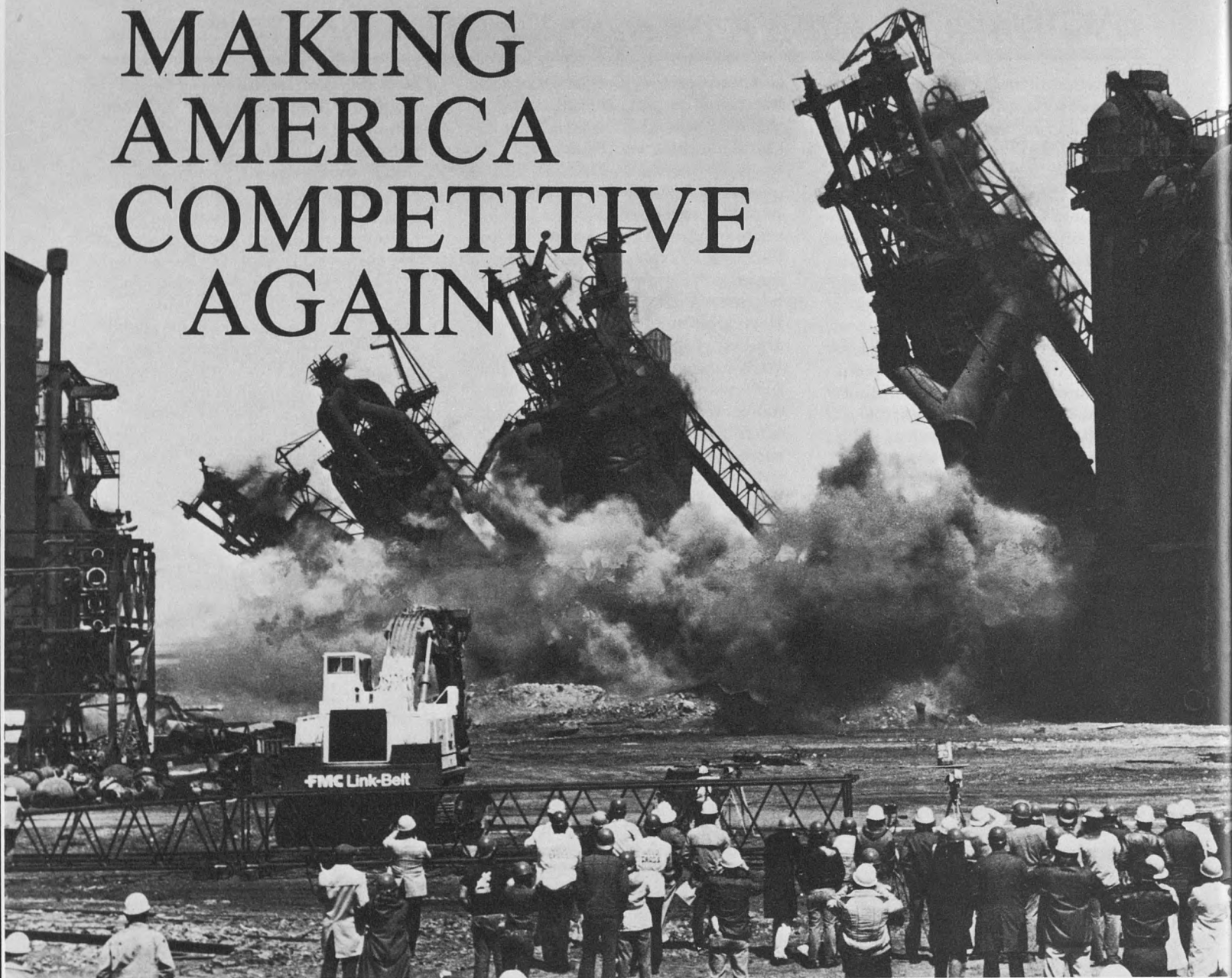
Four veteran blast furnaces are systematically detonated in rapid sequence at U.S. Steel's former Ohio Works in Youngstown to make way for further progress on a modern U.S. Steel Industrial Park. (Courtesy U.S. Steel Corporation)
