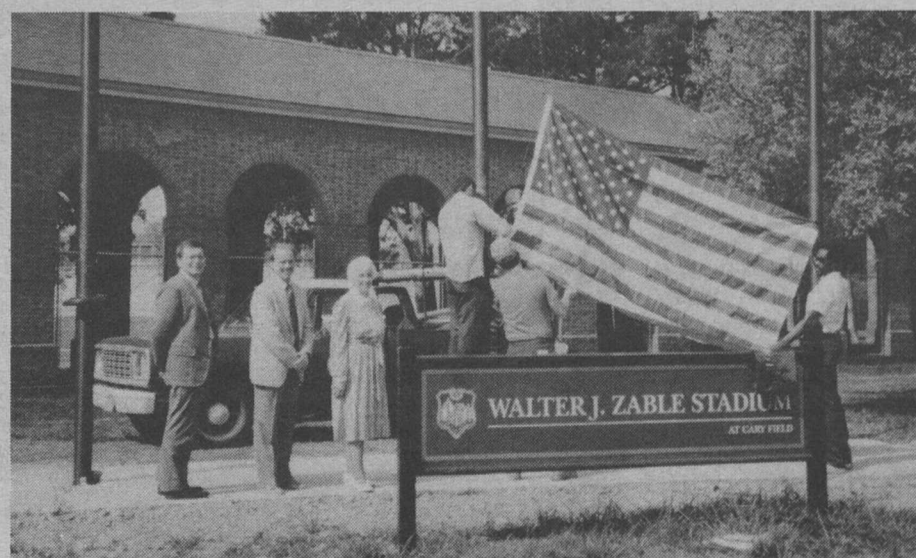
New flagpoles have been installed at the entrance of Zable Stadium, thanks to a gift from the Williamsburg chapter of the Society of the Alumni. Watching the installation by members of the College's facilities management staff are, from left, Barry Adams, executive vice president of the Society of the Alumni; John Rhodes '75, treasurer of the Williamsburg chapter; and Elaine Baker '49, chapter president. The flagpoles, which will prominently display the United States and Virginia flags, as well as a new William and Mary flag, were previously located in front of Blow Memorial Hall but recent renovations there necessitated their relocation.
