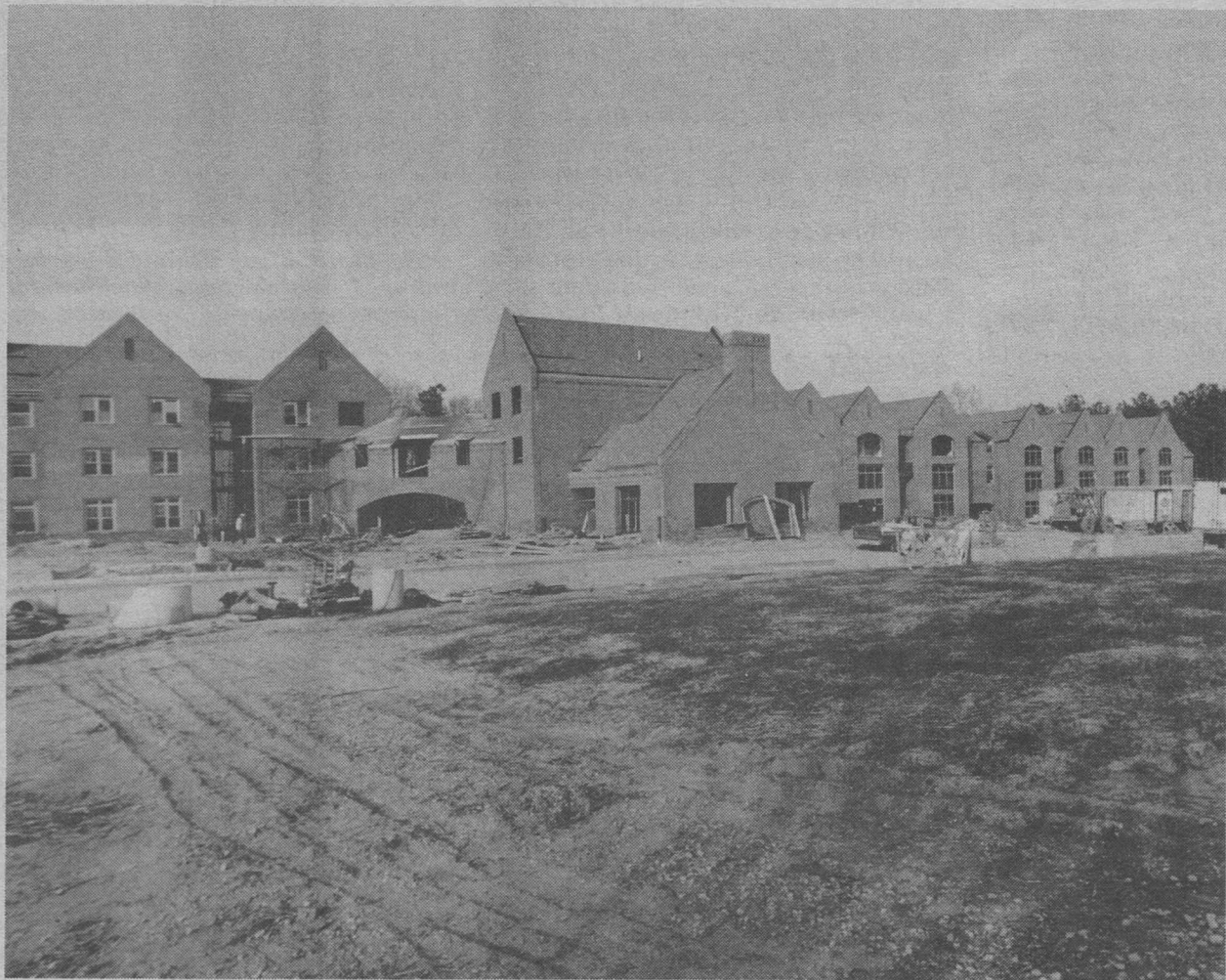
Now under construction, the $7.2 million graduate student housing complex will be ready for occupancy this fall. It will accommodate 240 students in two-, three- and four-bedroom apartments.
