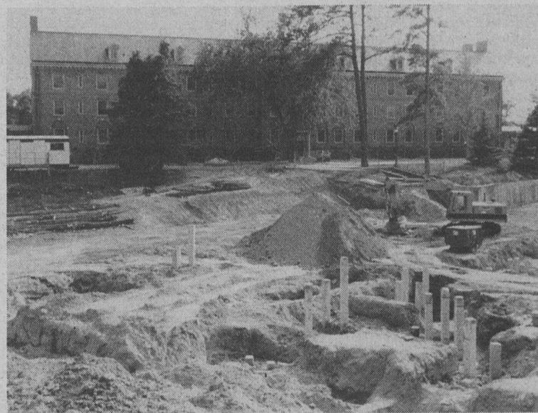
Ground was broken last spring for Tercentenary Hall, which will complete construction on the "Old Campus" established by the College's Master Plan in 1925. The four-story building will include instructional and research laboratories, administrative offices, departmental libraries and a large lecture hall on the ground floor to be shared among the disciplines. It is scheduled for completion in the fall of 1994.
