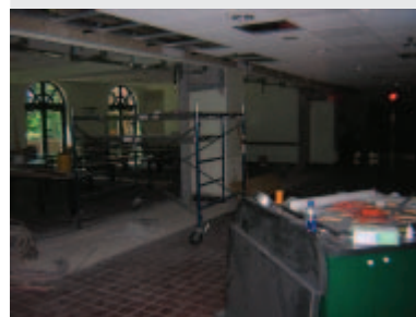
The UC saw the removal of several walls to make room for new drink and salad stations.
