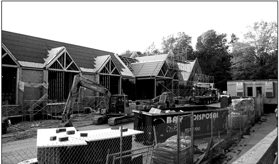
Construction continues on the Rec as the College creates a new state of the art facility.
