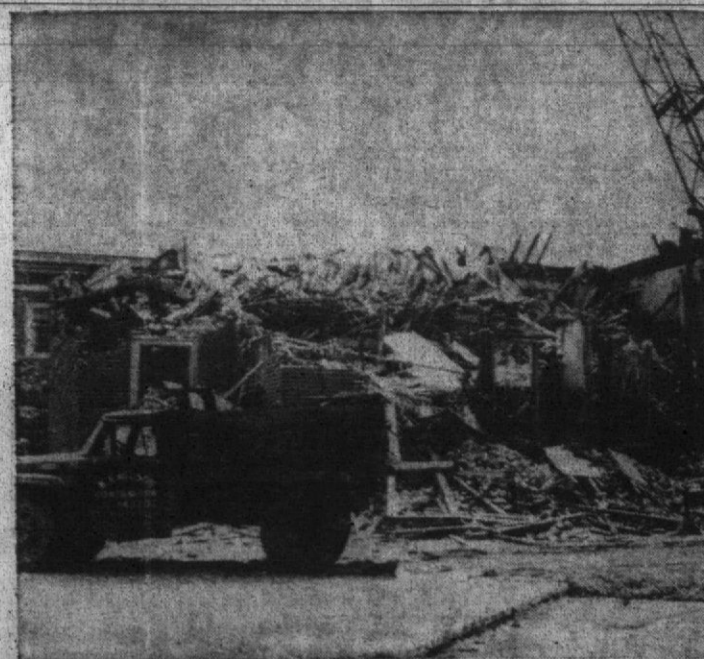
Old Talistero Hall, better known as the old fine arts building, is captured in its last days of existence. The Robert Andrews Hall of Fine Arts will replace the building which was razed this past summer. Photo by Dean Olsen
