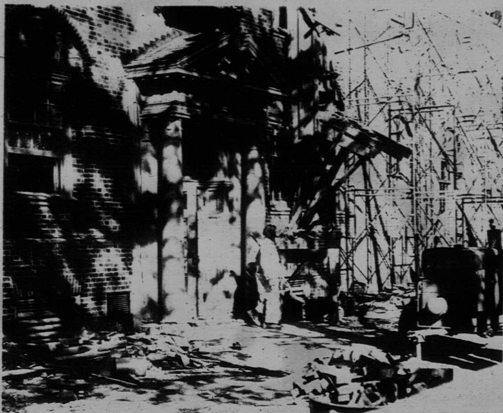
A workman exits from the Jefferson renovation project. Heindl-Evans, the contractor, notified the College two weeks ago that the building would not be ready for occupancy in January.
