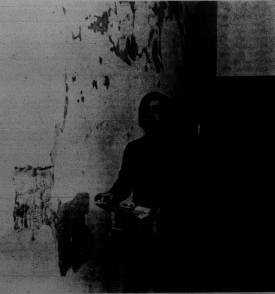
Missing paint and plaster in first north
