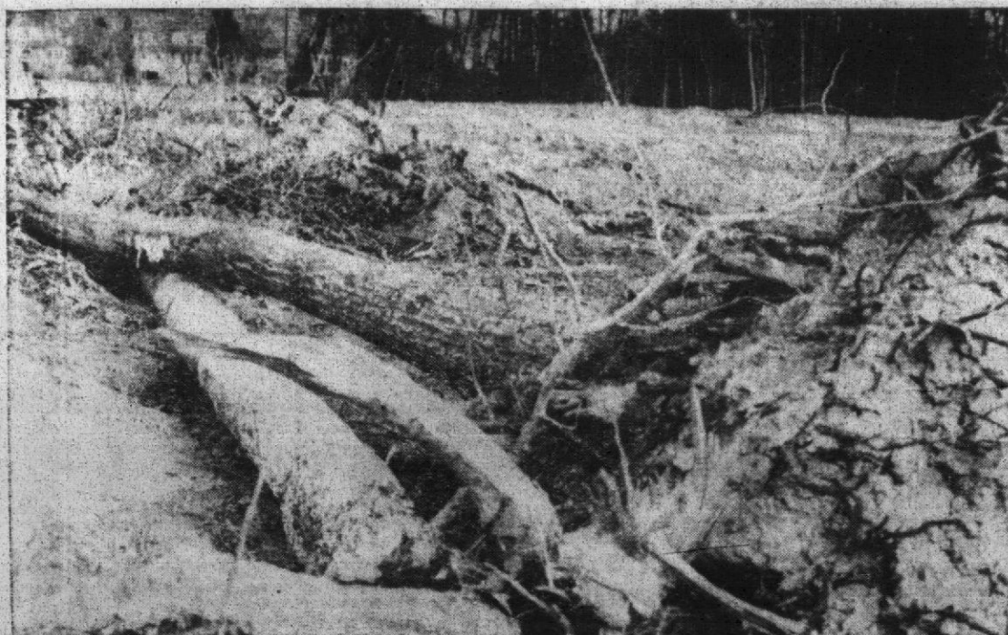
Initial clearing of wooded acres near Yates Dormitory provides for surveying and excavation.
