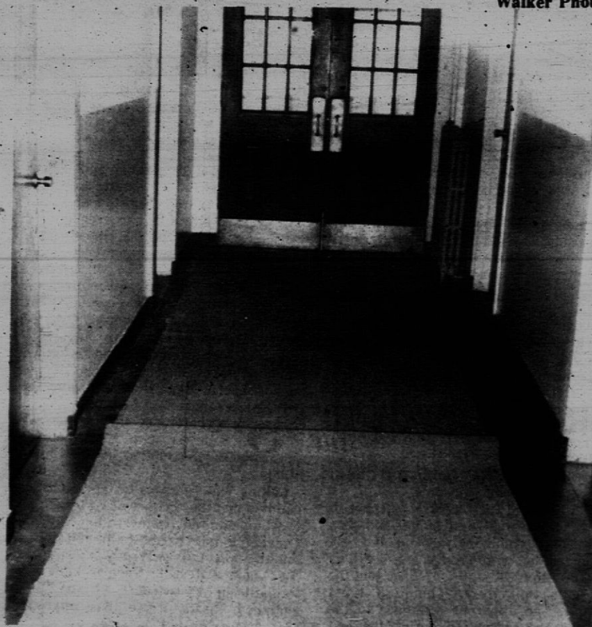
Improperly installed carpet causes danger to Hunt residents.
